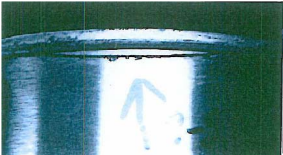
16 Pointer indicates a "knocked down flange".
